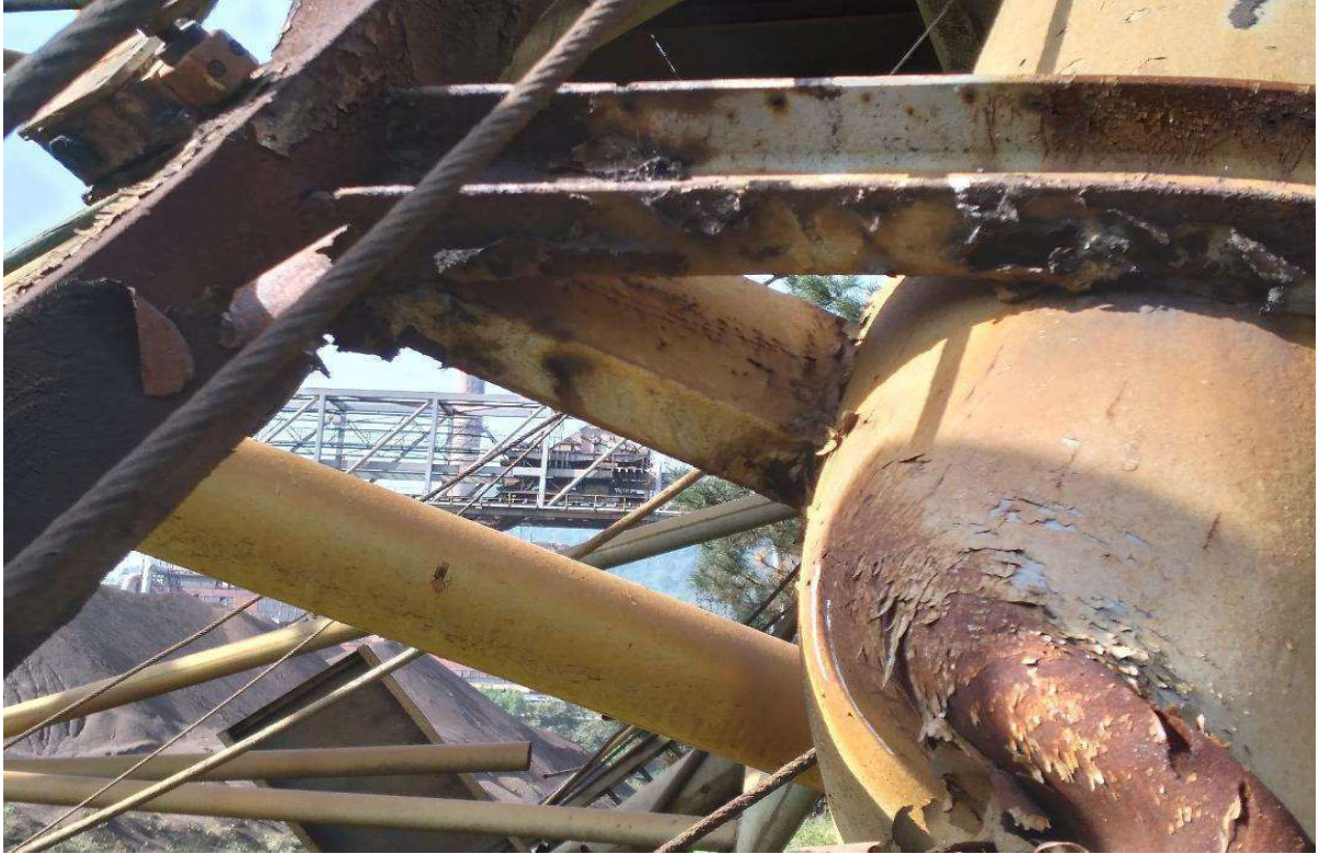
Figure 7. Detailed position of the small ductile breaks of a broken portal crane section
