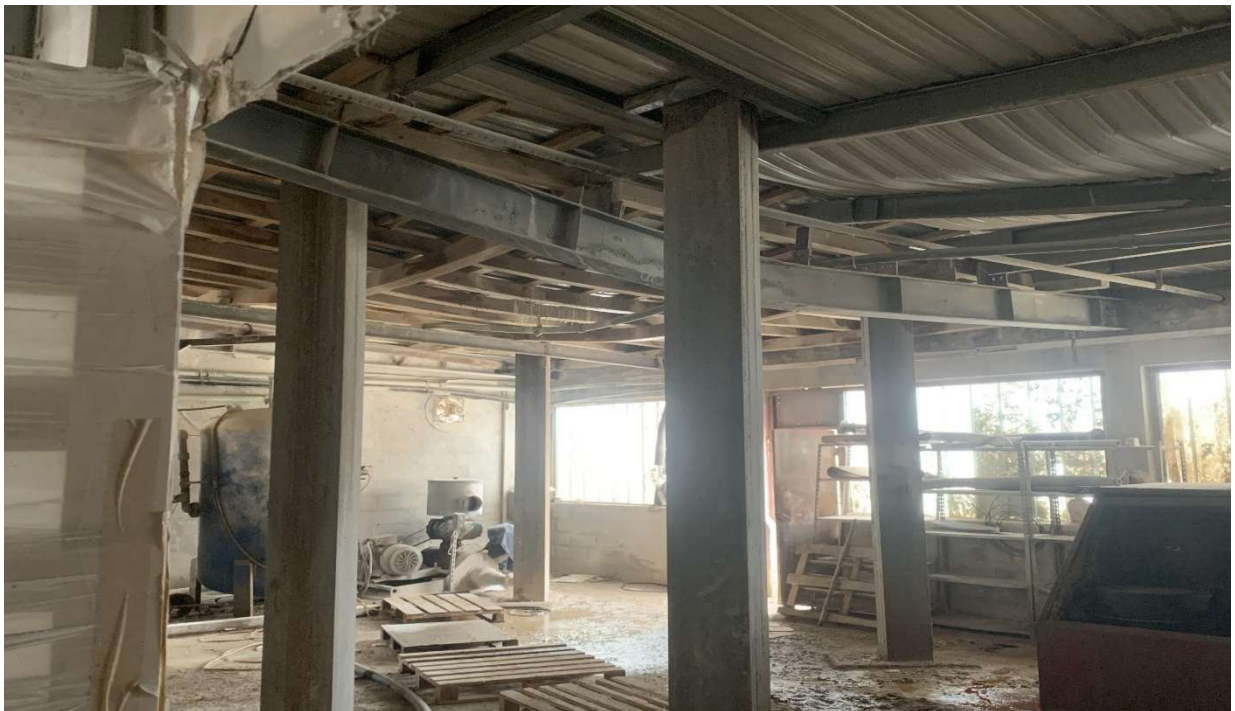
Figure 10. Detailed position of the wooden section supports to plastically deformed sections & roof
