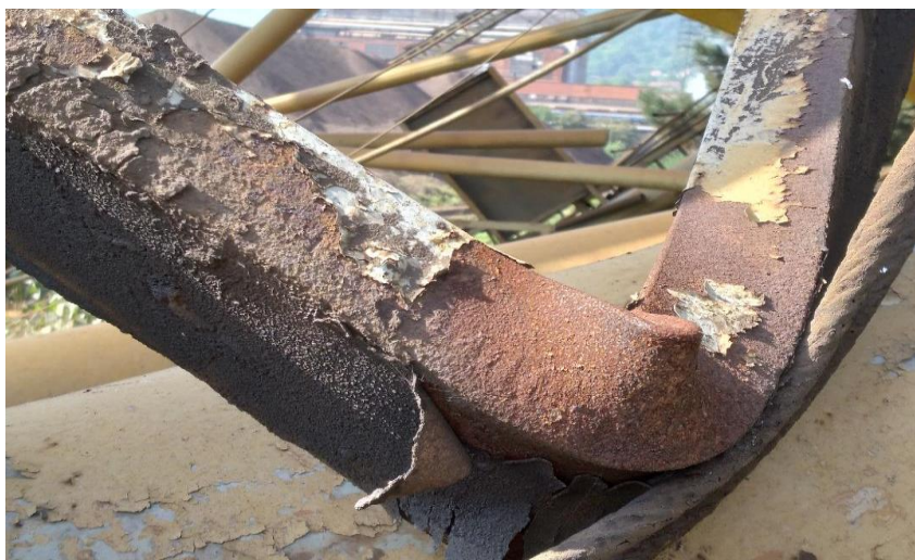
Figure 5. Detailed view of a severely plastically deformed (bent) section of a broken portal crane
