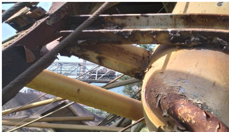
Figure 8. Detailed position of ductile fracture of a broken portal crane section
