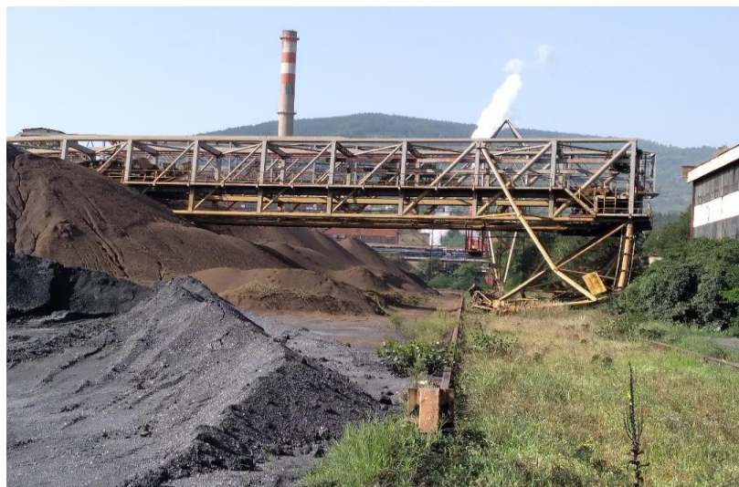
Figure 2. An example of the broken portal crane
