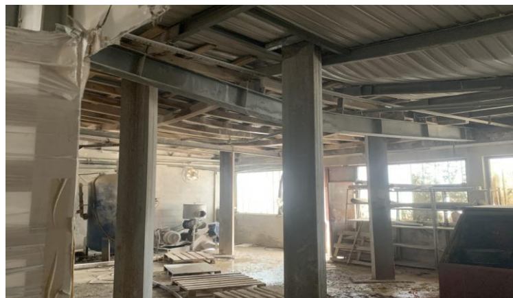
Figure 11. Position of the wooden construction supports to plastically deformed sections & roof
